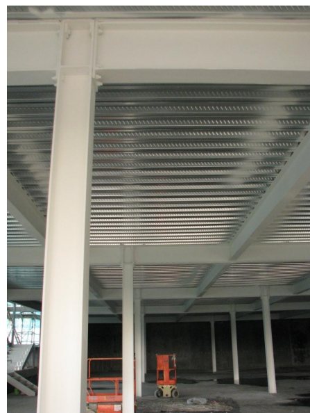
Freshly applied fireproofing coatings in a hospital construction. Credit: Altex Coatings Ltd.
